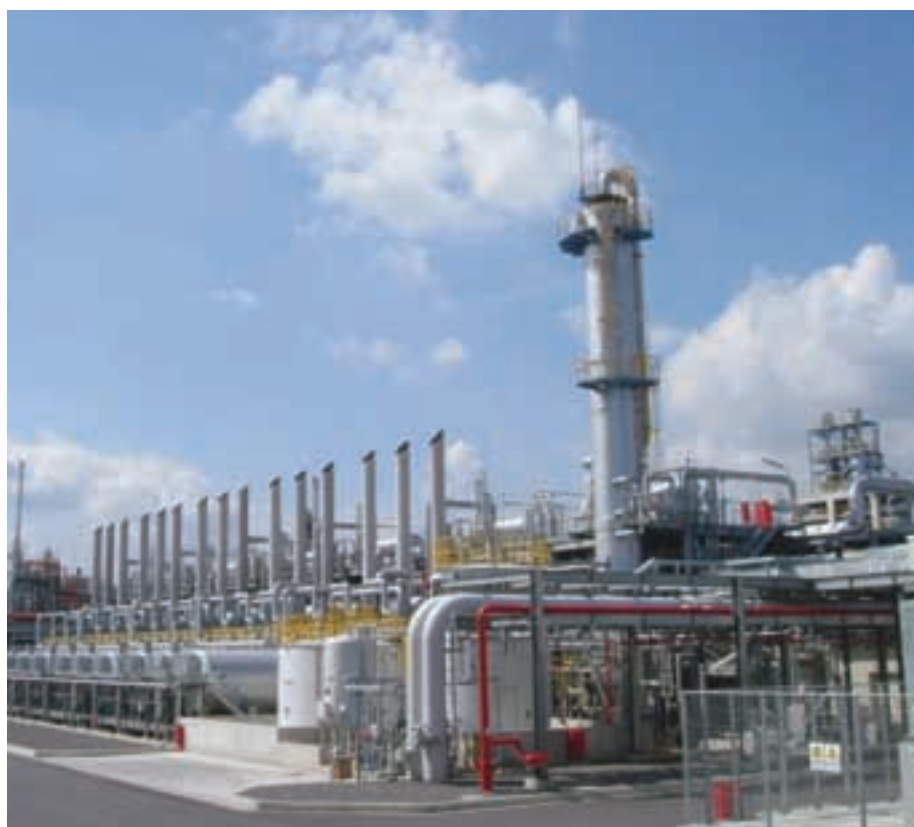
Manufacturing facility for acetate tow for cigarette filters in the Ohtake Plant
