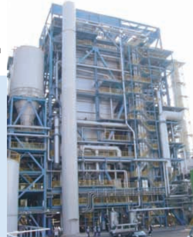
The Ohtake Plant's circulation fluidized bed boiler
